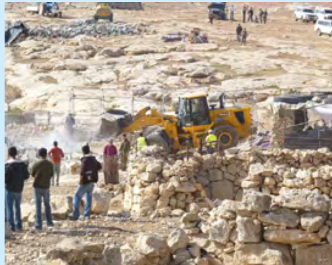
House demolition by the Israeli occupation forces in South Hebron. Photo by B'tselem.
