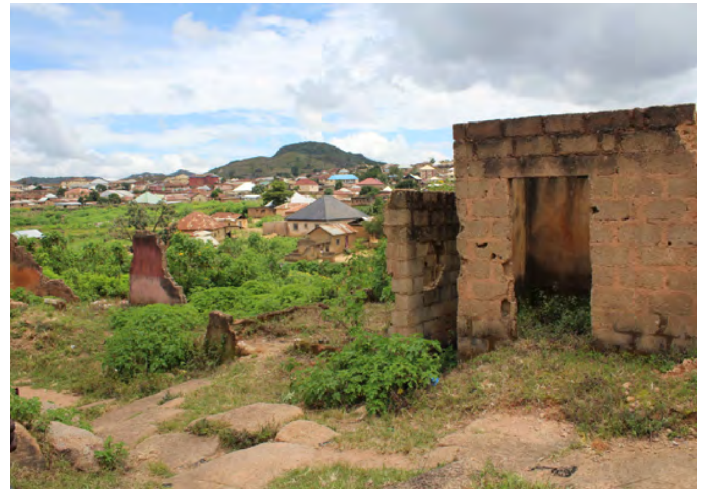
Burnt houses due to communal conflict in Angwan Damisa, Jos, Plateau State
